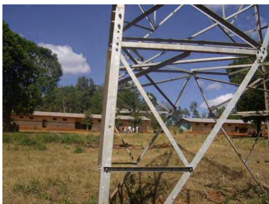
Electricity tower in school compound
