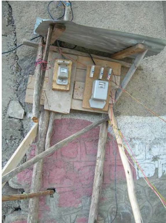
Figure 6.4: Electricity facility in Ethiopia (Source: Author)
